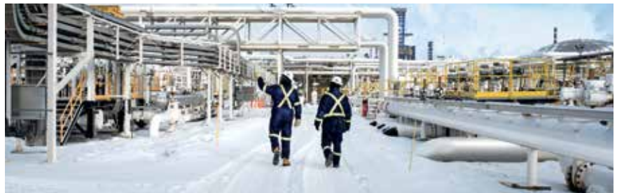
Variable speed drive electric motors at pump stations help to reduce the emissions profile of Enbridge’s liquids pipelines business.
